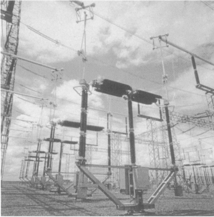
Figure 6-12: Special T-Circuit breakers used at Garabi Converter Station [ABB]
