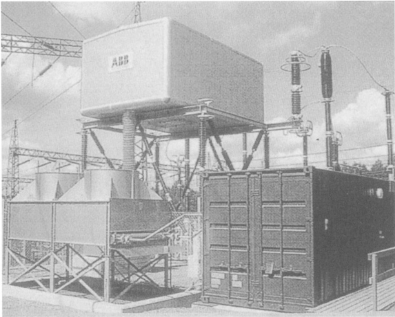
Figure 15-4: Outdoor valve in operation at Konti-Scan I station [ABB]
