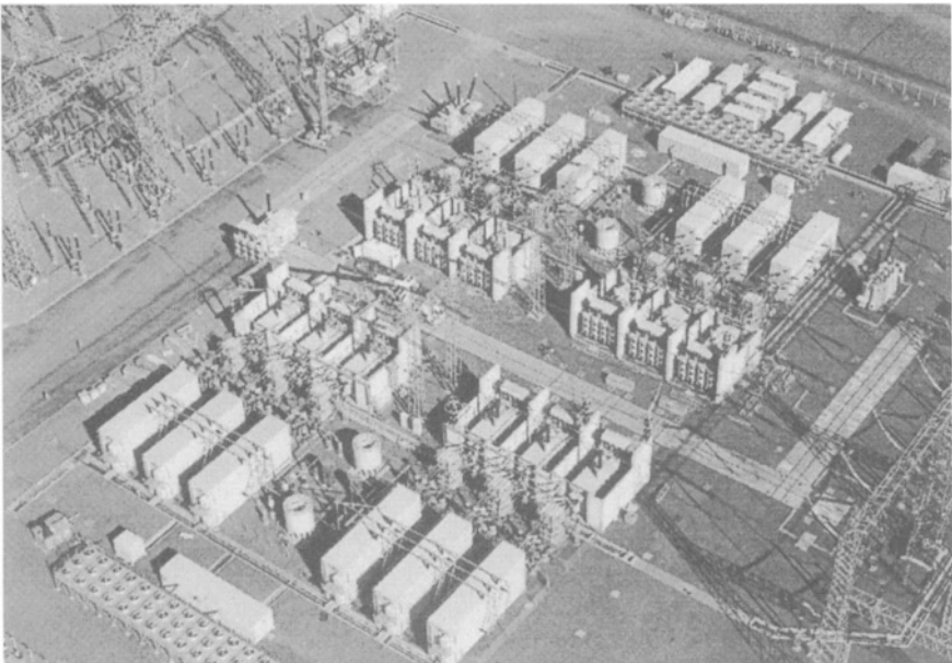
Figure 6-11b: Aerial view of CCC at Garabi [13, 14 and ABB]
