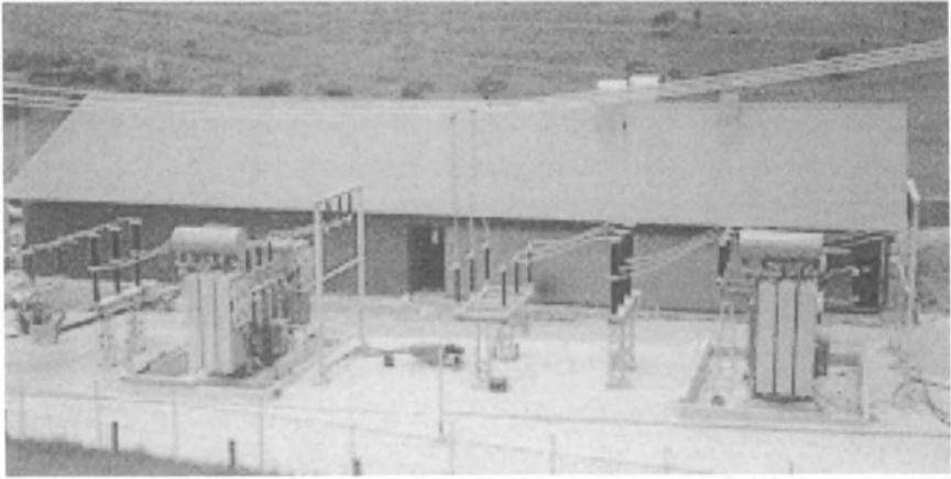
Figure 8-15: One of the Directlink converter stations [ABB]
